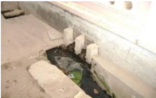
Existing Sewerage system
