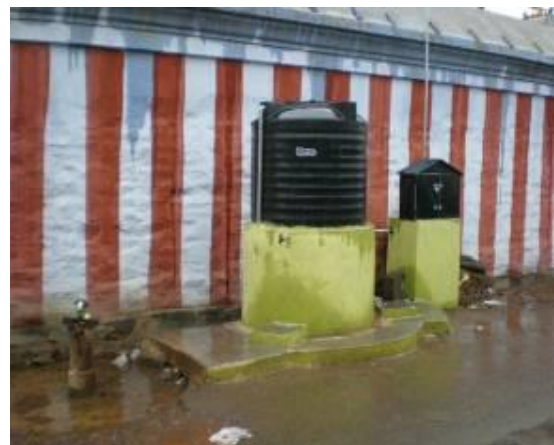
Water distribution tank
